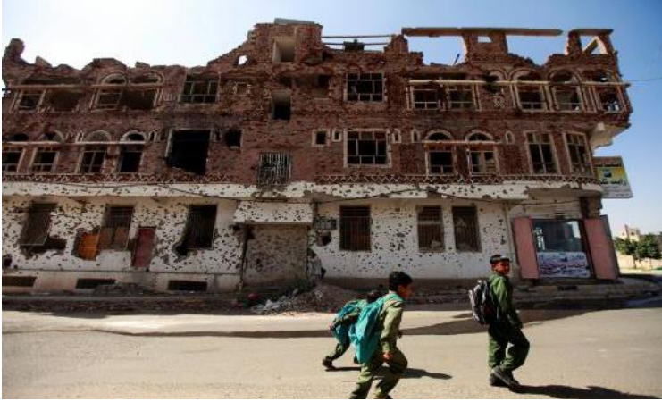
Boys on their way to school walk past a building damaged during protests and clashes in 2011 in Sanaa, December 17, 2013.
